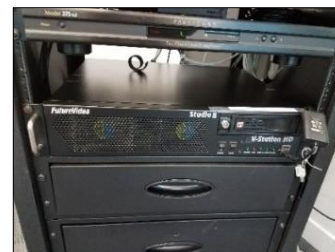
V-Station HD Studio8 in SWDS' 19" Rack
